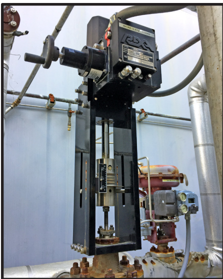
Condensate Level Control
