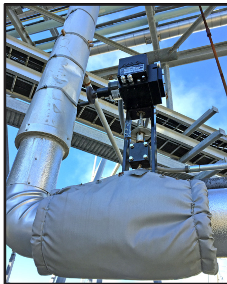
Steam to Fuel Gas Heater
